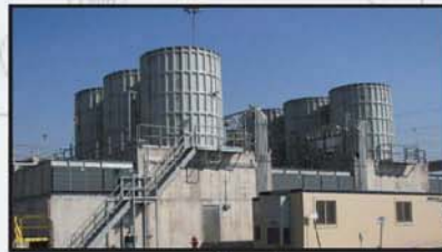
Blast furnace cooler
