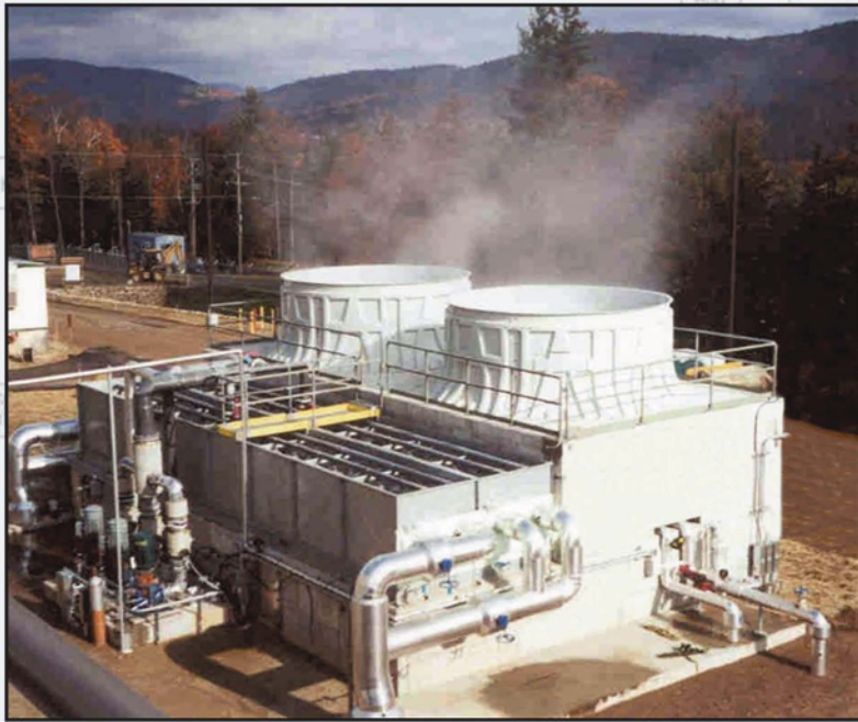
Auxiliary water cooler
