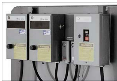
Starters shown mounted & wired.
