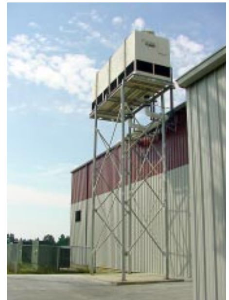
A TC-405F cooling tower cell mounted on a 30' stand. The stand height was required because the pump tank is mounted inside the building on a mezzanine. You'll notice that the stand is a little wider than the tower to provide a broader base for support. A well anchored pad was required to offset the wind loading force on the tower.
