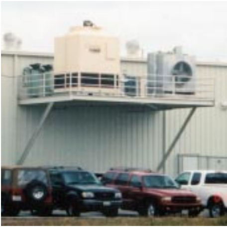
A unique tower stand expands parking capacity while holding this ADVANTAGE tower system in Northern California. The picture shows the cantilevered support holding TC-135F and Marley tower cells.
